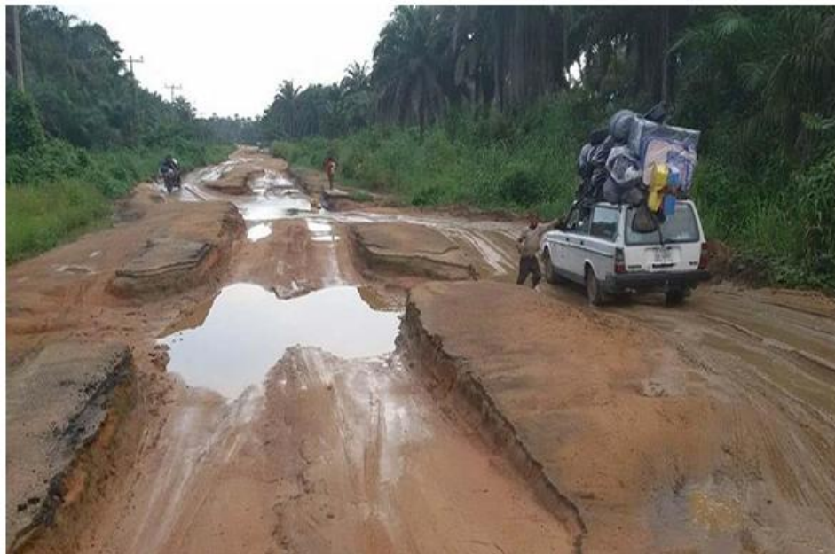
Fig. 2: Typical Deplorable Road Network in Akwa Ibom State
