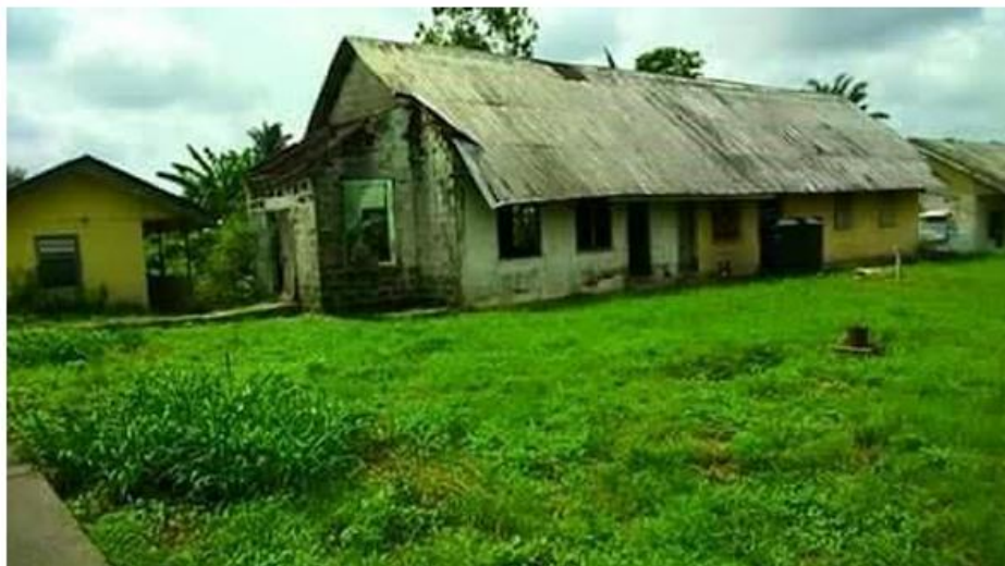
Fig. 1: Typical Dilapidated Health Centres in Akwa Ibom State
